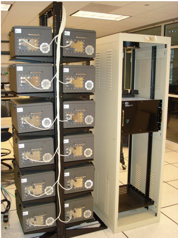
Fig. 2. Assembly and connection of the shielded enclosures and RF switch.
